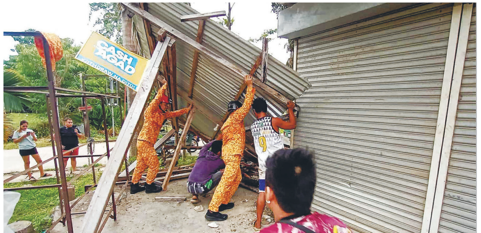
Firefighters and residents fix a damaged roof in Baganga town, Mindanao. - AFP/IC/BUREAU OF FIRE PROTECTION REGION 11
