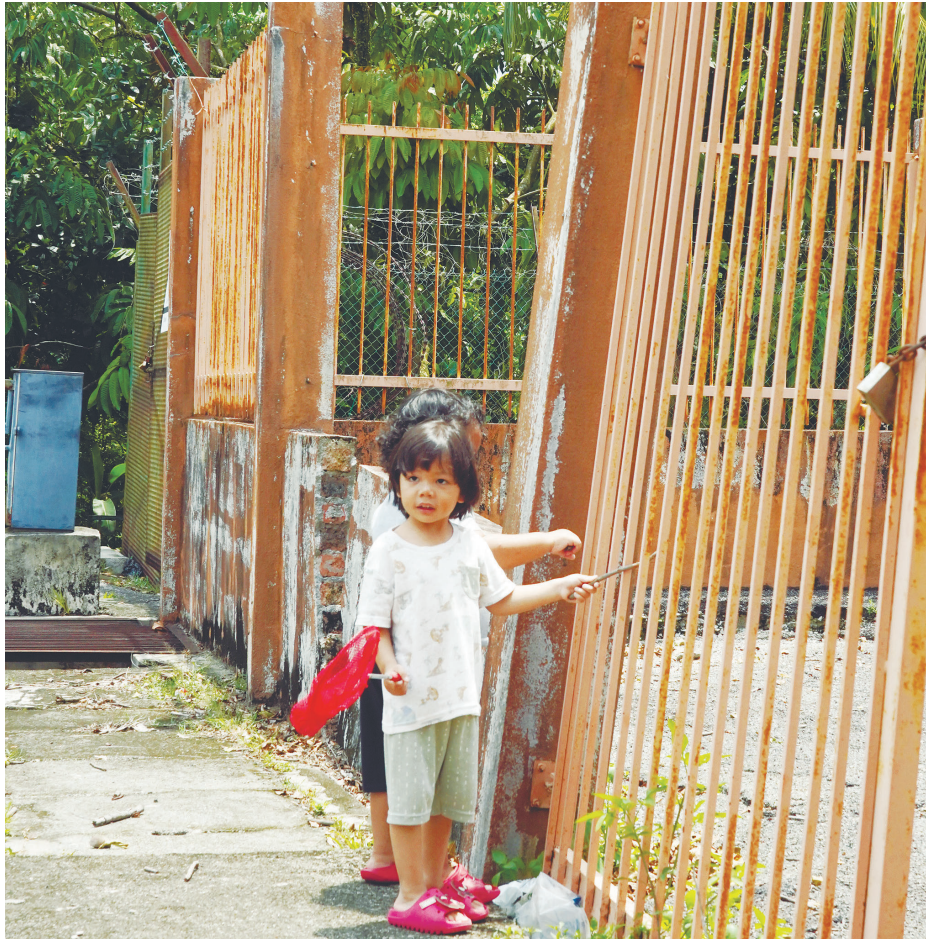
Che Khairil said structural collapses often stem from basic technical errors that could easily have been prevented with professional input. – AMIRUL SYAFIQ/THESUN
