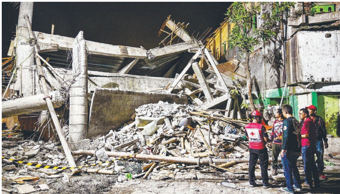
Rescue personnel inspecting the site after the building collapsed. – AFP/PIIC
