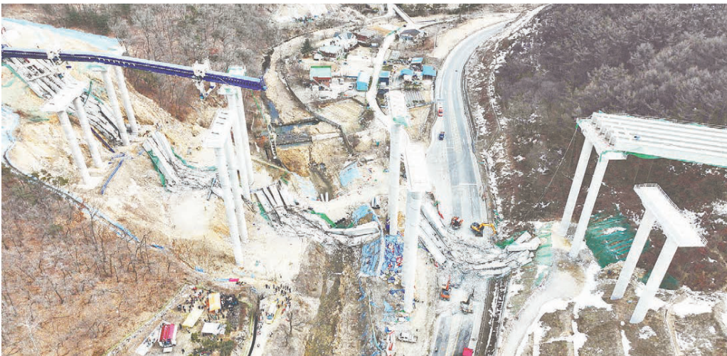
Rescuers searching for missing workers at the construction site in Anseong yesterday. - AFP/FPIC
