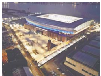
An aerial view shows Everton football club's new stadium under construction at Bramley Moore Dock in Liverpool. – AFP FILEPIC
